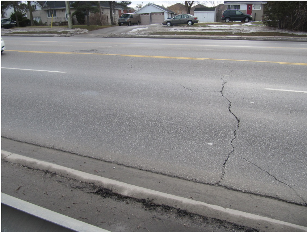
Photo 3: Transverse and meandering cracking on Coleraine Drive
