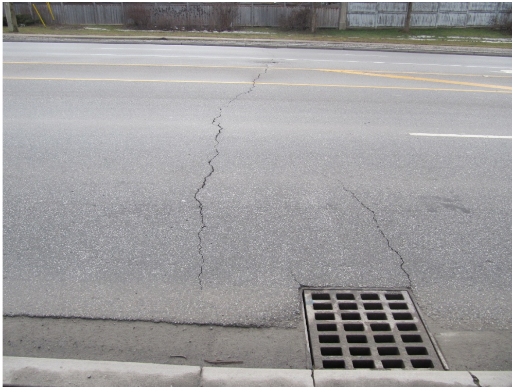
Photo 1: Transverse cracking on Coleraine Drive
