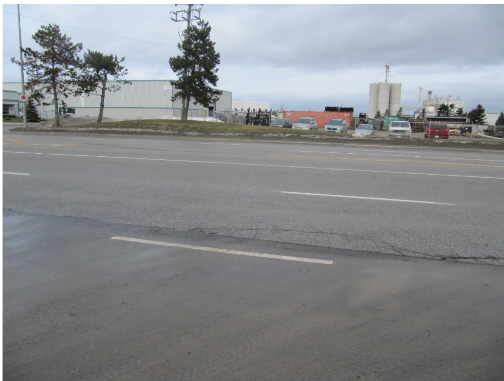
Photo 2: Patching and fatigue cracking on Coleraine Drive
